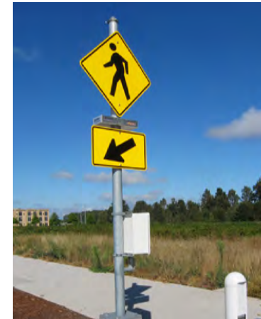
Rectangular Rapid Flashing Beacon example image
